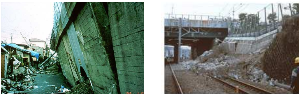
Figure 12. Examples of seismic damage of conventional reinforced concrete walls
